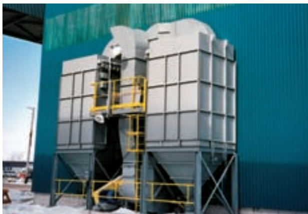
Two TubeJet collectors remove limestone dust from a utility scrubber dumping station. Each collector handles 11,000 ACFM.
